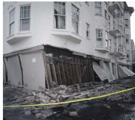
“Soft story” buildings, typically with parking on the ground floor, like the one pictured here, are common throughout the Bay Area and are particularly at risk when exposed to strong shaking (USGS photo).
