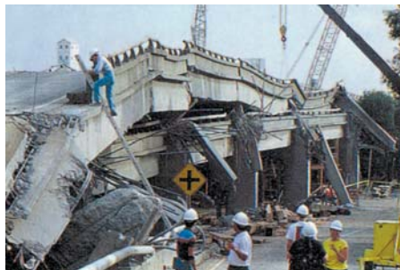
Big earthquakes will damage roads and bridges , causing accidents and traffic jams and making it harder for rescue workers to help injured people. Commutes will be affected for days, weeks, or even months (USGS photo).
